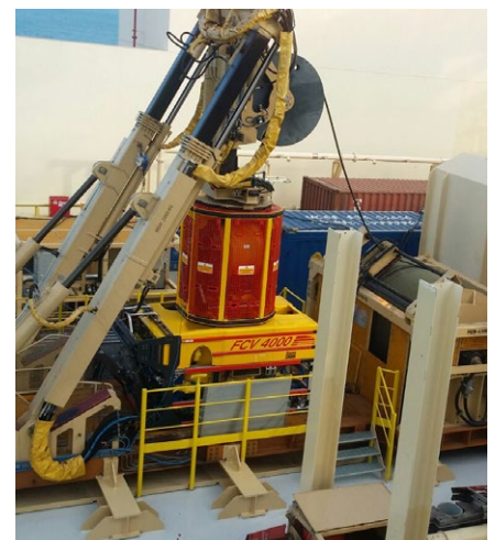
FCV 4000 installed onboard Samsung 96K Drillship
